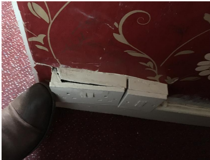
One of many loose electrical fittings
