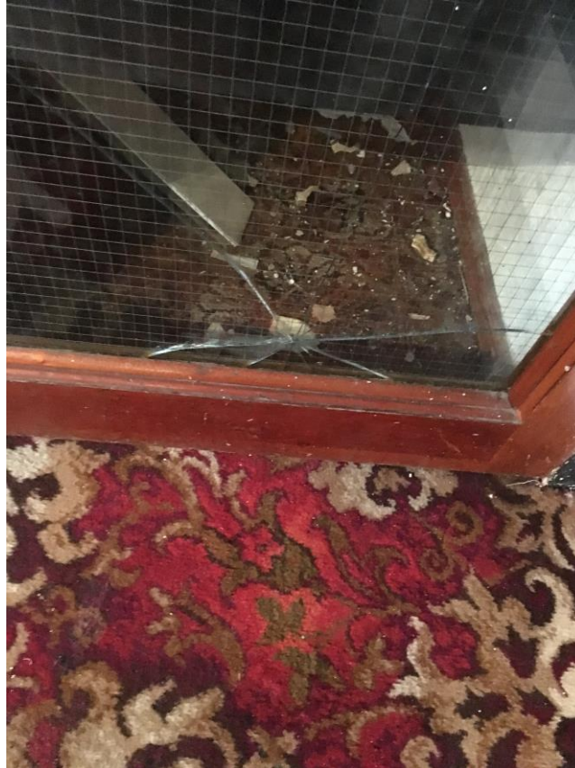
One of many cracked in glass panels throughout the hotel
