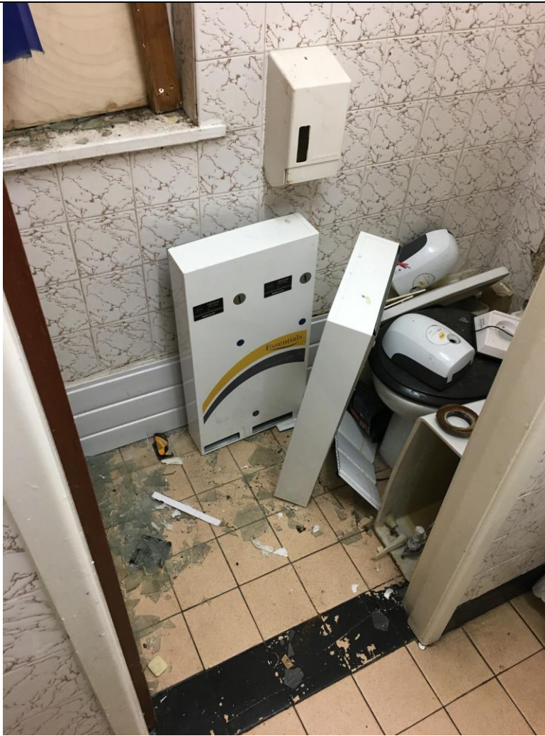
Ground floor toilet, not cordoned off to public/residents
